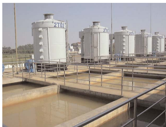
Nam Du Water Treatment Plant in Hanoi
