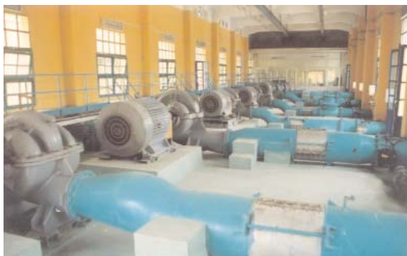
Treated Water Pumping Station in Hai Phong
